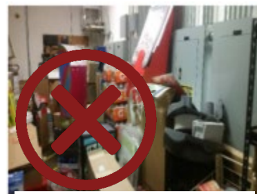
Do not block electrical panel
