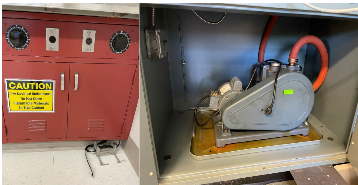
Figure 5: Live outlet cabinet for a vacuum pump outside (left) and on the inside (right).
