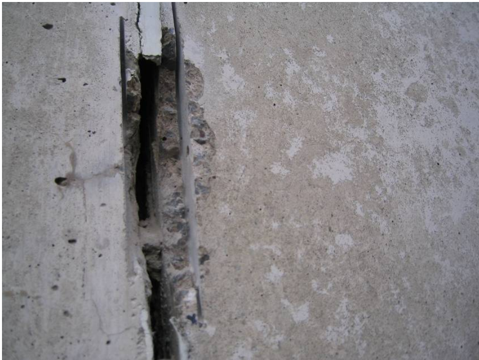
Photograph 4 Example of Channel Cut, Approximately 1/4" Cut from Caulking
